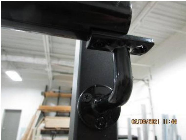
Photo No. 4 Bracket Connection - Post Mount
